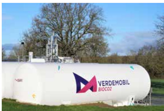
GAZTEAM BIOCO2 (79) | ©VERDEMOBIL BIOGAZ
