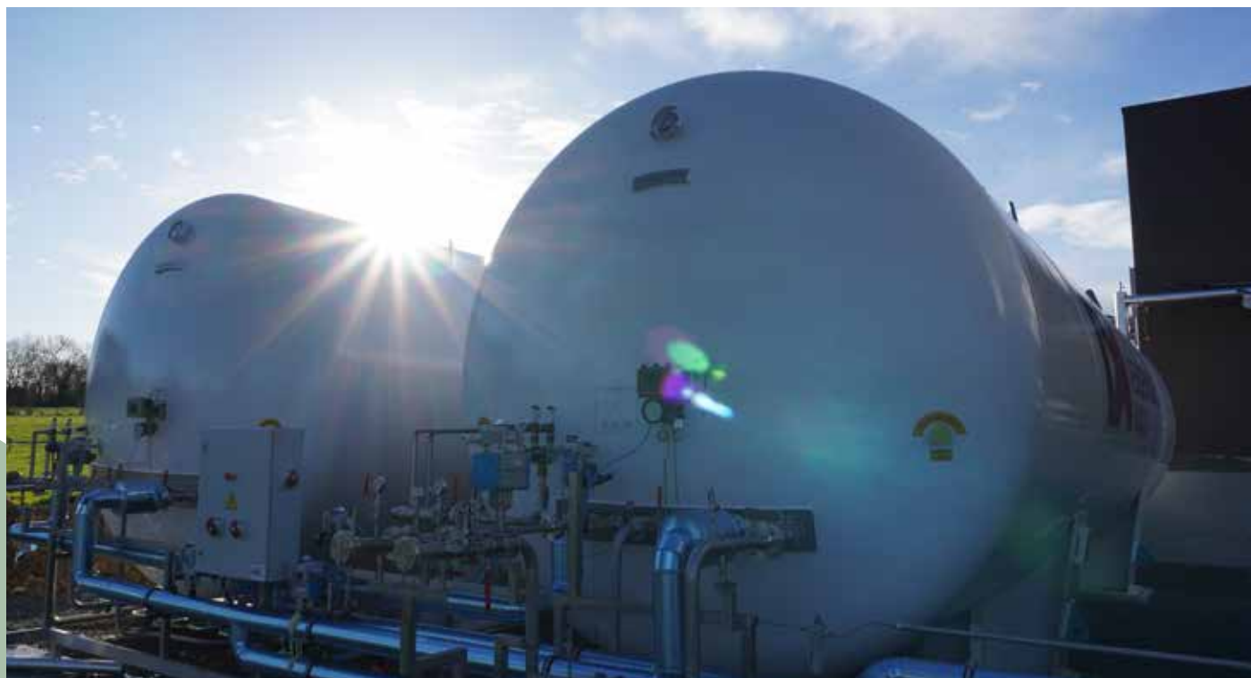
GAZTEAM BIOCO 2 (79) | ©VERDEMOBIL BIOGAZ
