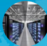
Data center DENMARK
